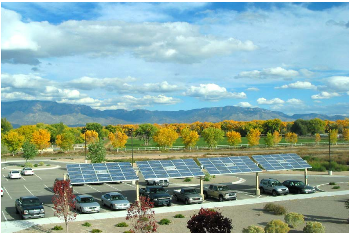
Visually integrated PV array and shade structure
